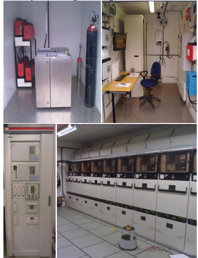
Figure 2. Battery and hydrogen storage system (top left) are separated from the various controllers, converters and other electrical equipment (top right). The RD 2 is connected to a medium voltage substation refurbished with a multi-vendor IEC 61850 (bottom left and right)
