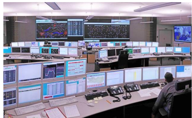
Figure 1: Control centre at the KELAG Netz GmbH
