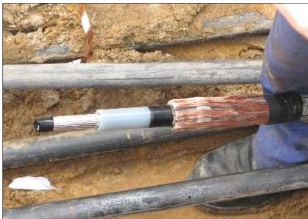
Image 1 – MV cable prepared to cross-bonding joint installation (cooper return conductor being separated)
