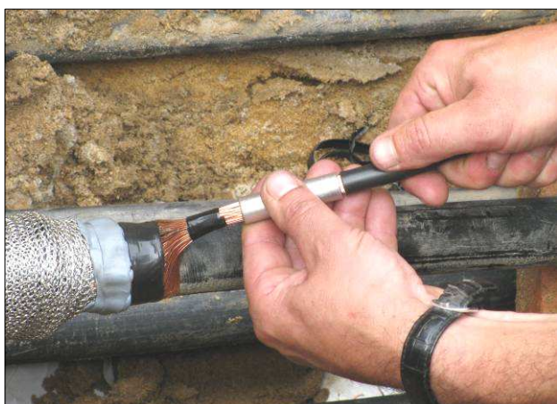
Image 2 – one phase return conductor pulled outside in order to connect it with other phase return conductor (crossing)
