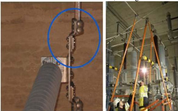
Fig. 7: Left: Detail of Disconnecting link; Right: Crew for live disconnection/reconnecting in action
