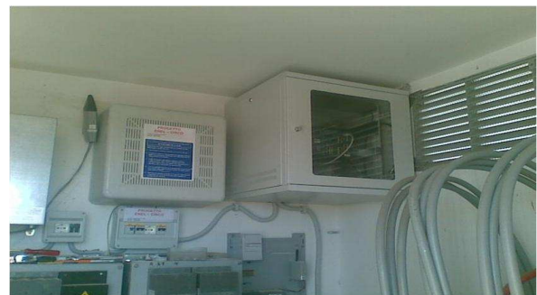
Figure 9: Secondary Substation Box
