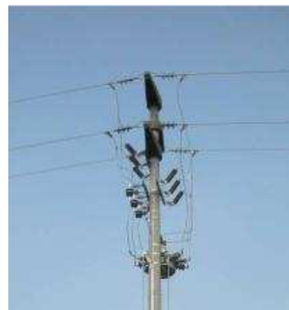
Figure 6: installation of an outdoor FPI on a pole installed switch disconnector
