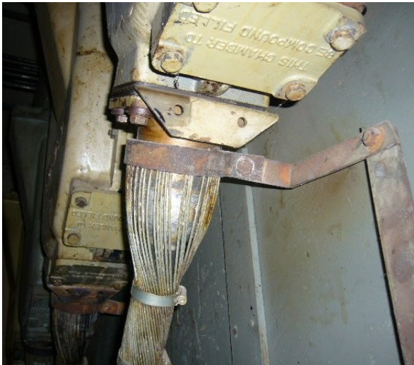
Figure 3. Example of poorly terminated cable sheath and steel wire armours.
