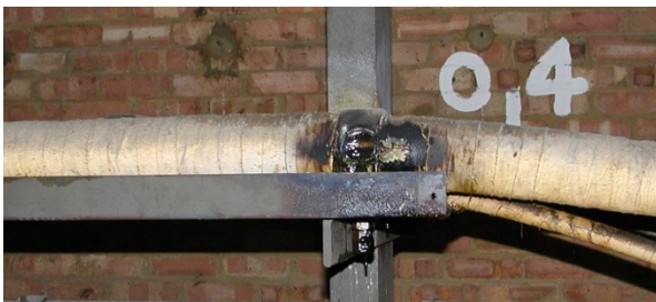
Figure 4. Cable damage due to poor sheath termination.
