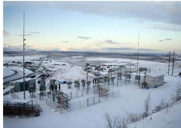
Picture 3. LKAB SVC system
