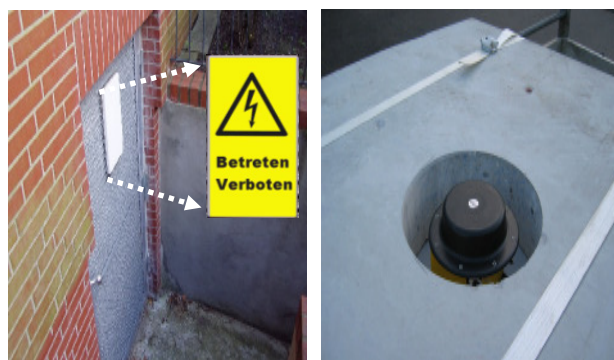
Fig. 7: Door sign antenna Fig. 8: Roof antenna without GRP cover
