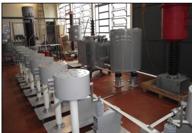
Figure 3: The transmission system built for the tests.
