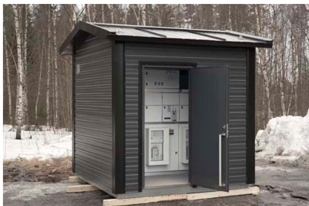
Figure 3: Ground mounted vacuum circuit-breaker application with one incomer and two outgoing feeders ( Recloser Station ). The network is either an overhead or a cable network.
