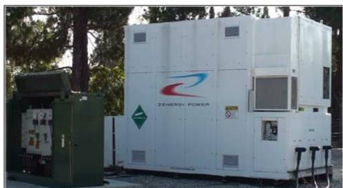
Figure 2. The CEC FCL installed at the SCE Shandin Substation in San Bernardino, California, USA.
