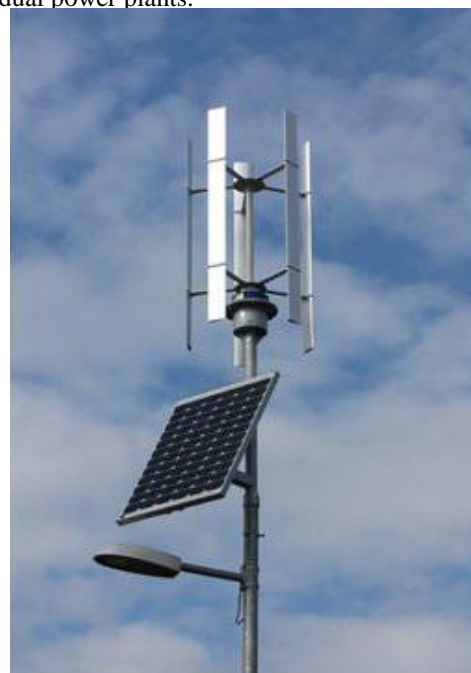
Fig. 1 Picture of half of the hybrid power supply system
