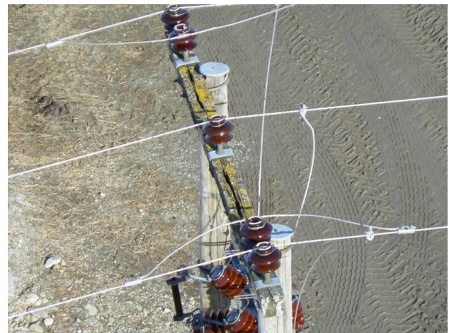
Image 1 Photo taken from helicopter – the cross arm is damaged by rot
