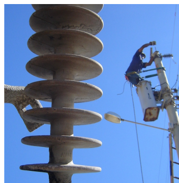
Figure 1 - Insulator from coastal area
