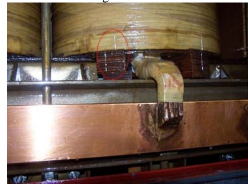
Bottom of phase B, low voltage side, after shock
