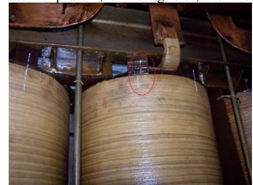
Top of phase B, low voltage side, after shock
