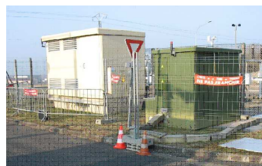
Figure 1: Transformer and load in the substations
