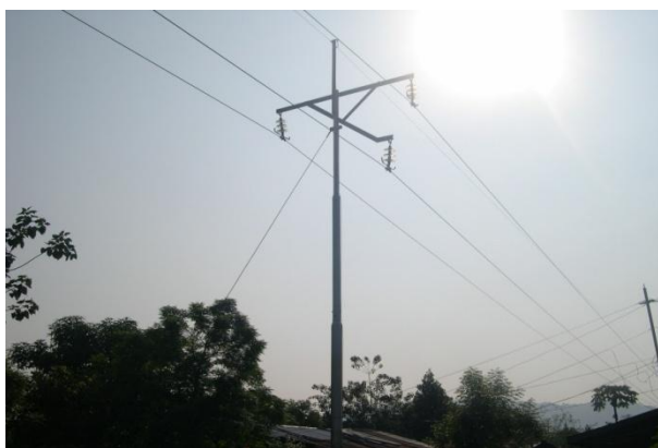
Fig.1(a). Distribution Line Photo
