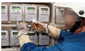
Figure 6 – First meter installations by Endesa
