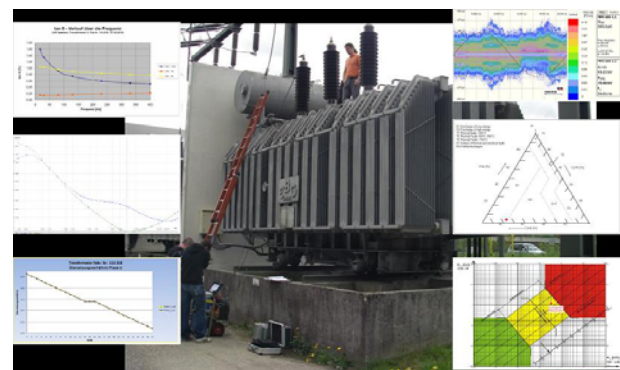
Figure 1: Transformer Onsite Measurement
