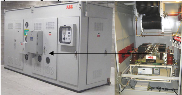
Figure 5. 10 Mvar capacitor bank and detailed view of switch.
