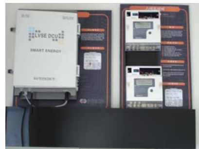
Figure 7. Installed Smart Meter and DCU
