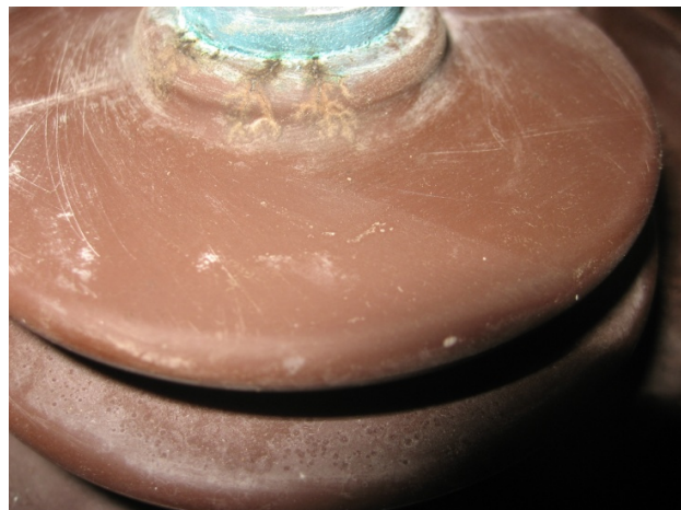
Figure 2: degradation due to tracking current on insulating parts
