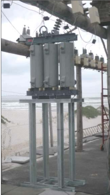
Figure 4. Outdoor Testing of dry-type pole mounted transformer (from LV side). The installation is placed around 30 m from the Atlantic Ocean in Western Cape of South Africa
