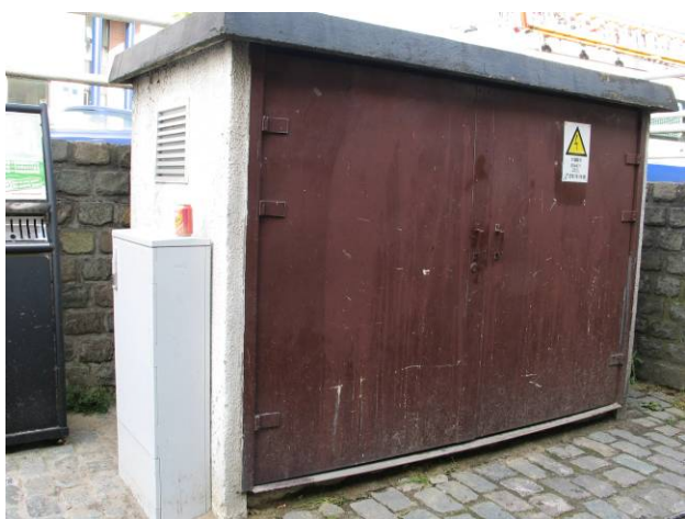
Figure 1: Substation at Waterloo – Cat 2 - Small standalone premise (compact substation) made of concrete with metallic doors rather exposed to weather conditions, with dark a roof
