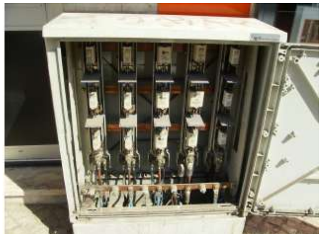
Figure.11: The typical street LV cables distribution box
