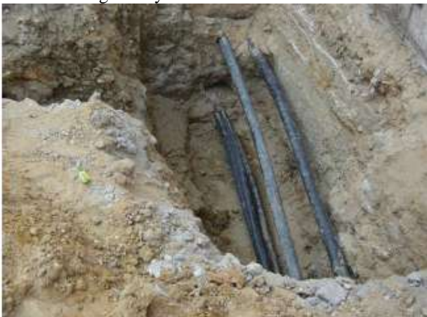
Figure 8: An open ditch showing a 10kV underground cable and some LV cables under a sidewalk.
