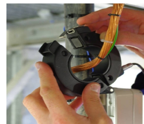
Figure 4. Connection of Current Transformer onto cable earth strap for online cable PD measurements
