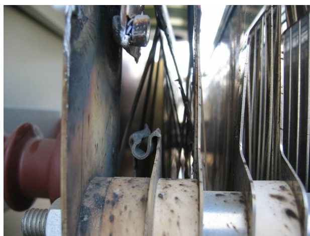
Figure 2: Failure of NGR caused by thermal overload [2]
