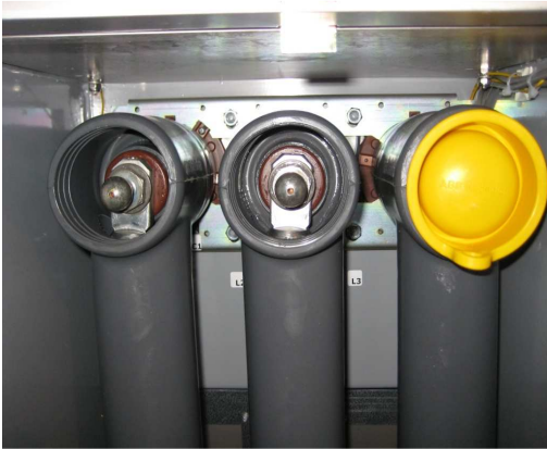
Figure 2: Conventional cable test interface on 12 kV cable connector in Xiria
