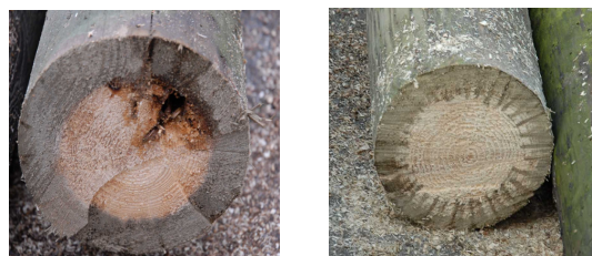
Figure 3: Comparison between the Polux measurement, the decay presence and micro-drilling method. Decayed pole on the left, sane pole on the right.
