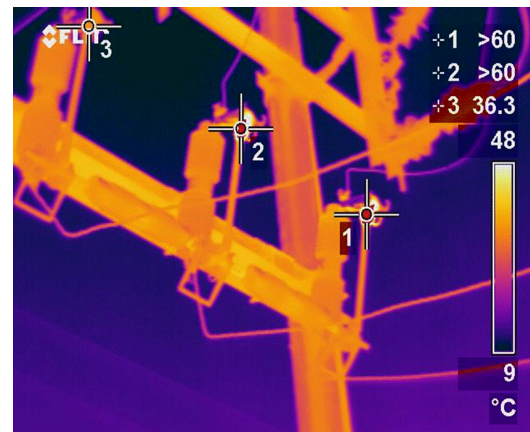
Photo 02: Hot-Spot Detection on EDO Fuse Assembly
