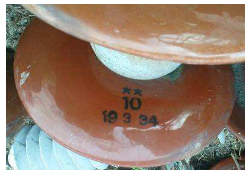
Photo 03: Use of Porcelain Insulators from 1934
