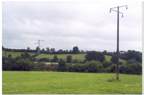
Fig. 4 Siemens 38kV Steel Tower/Wood Pole Line
