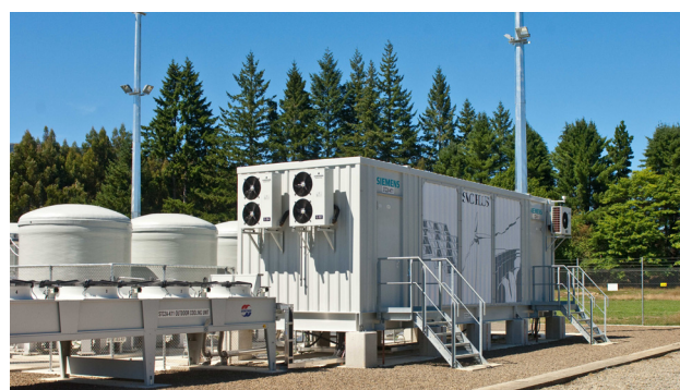
Fig. 2: View of one of the two SVC PLUS systems ( \pm 50 MVar) installed at Kikiwa, New Zealand
