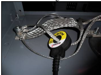
Figure 9 Permanent HFCT inside of cable box.
