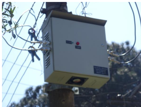
Figure a2 –PVRLVN Installed at the Training Center of AES Eletropaulo
