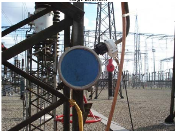
Fig. 5 - Partial discharge measurement in 345 kV substation – Detail of the high frequency CT applied to the grounding conductor.
