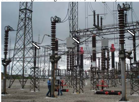
Fig. 4 - Partial discharge measurement in 345 kV substation in ZnO surge arresters.
