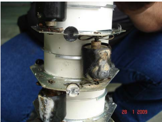
Fig. 12 – Damaged grading condensers inside arrester, possible cause of partial discharges.
