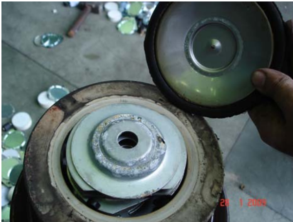
Fig. 11 – ZnO arrester after opening. Some white corrosion can be seen in metallic parts.
