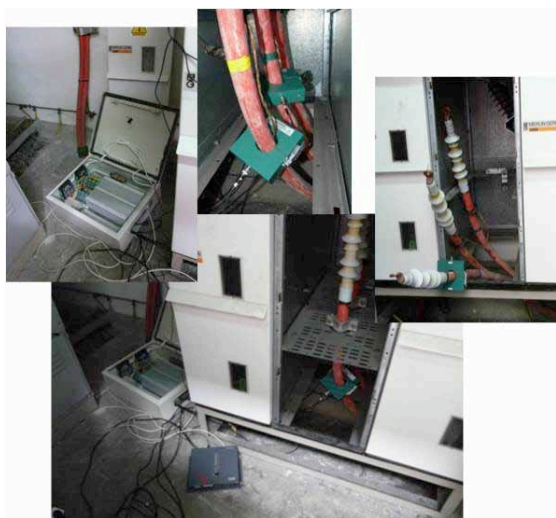
Figure 8. Data acquisition system installed in a MT substation
