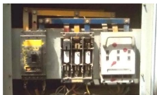
Figure 3: Photo of cubicle 2
