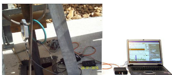
Figure (2) On-site Measurement set-ups for PD detection using HFCT for 66kV – XLPE Insulation
