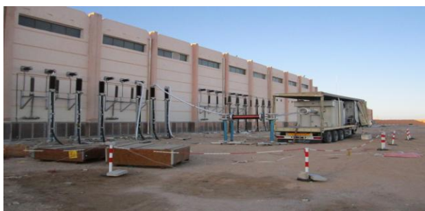
Figure (1) Frequency tuned resonant test system (20 Hz -300 Hz) - connected with XLPE- cable circuits 66 kV
