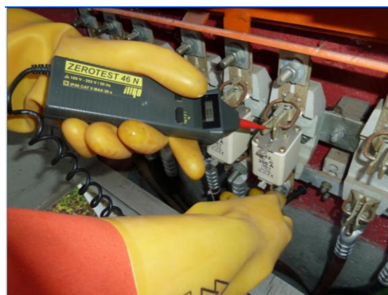
Fig. 2: measuring instrument Zerotest 46N for short circuit impedance (phase-earth) measurement, practical real measurement
