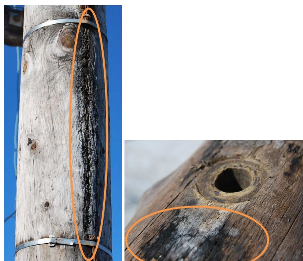
Fig 3: Tracking observed at KIPTS: a) in insulation coordination gap (left), b) at uncapped insulator without conductive plate (right)
