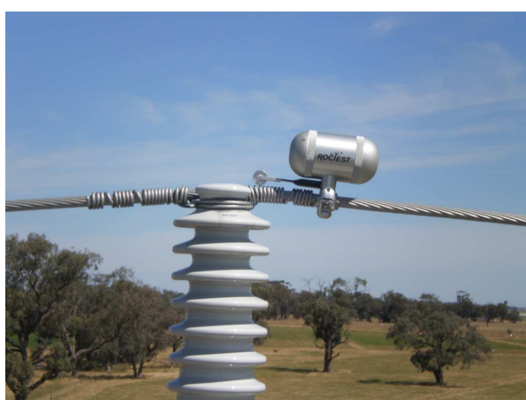
Figure 2. View of recorder installed on vertical insulator on concrete Pole 314
