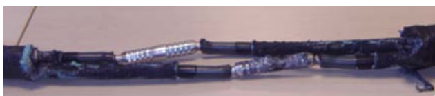
Fig 2. Joint failure caused by thermo-mechanical forces.
