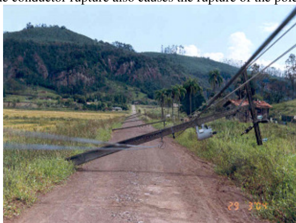
Figure 4 - Windstorm - Rural area
