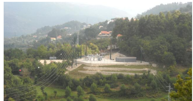
Fig. 10 - Caniçada substation - general view
