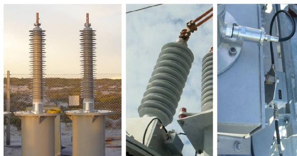
Figure 5: Two 123kV oil-air RIS bushings at KIPTS test station (SA) (left); a 72.5kV RIS bushings operating at Axpo's substation Grynau in Switzerland (middle) and its connection to the monitoring system (right).
