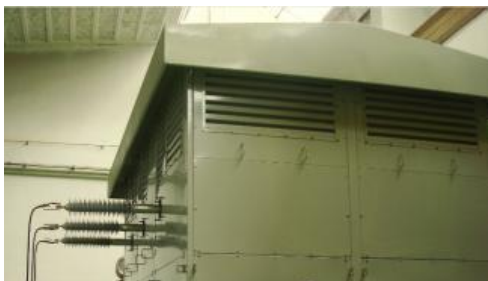
Fig. 4: HiDry 72 transformer mounted in outdoor enclosure
