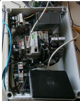
Fig. 4 - Sigma Tele-control box enabling the automation of the shedding process by the customer facility
