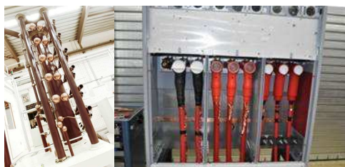
Figure 6: Test object with 3 types of cable connectors in Prof. Ir. Damstra Laboratory.
