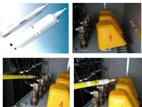
Figure 5: Volt Stick in operation on a transformer.
