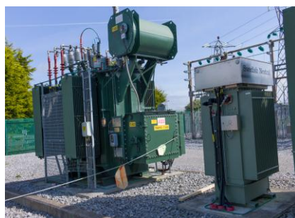
Figure 2 A modern fast tuning solid core arc suppression coil (right hand of picture) forming the high voltage part of the GFN system
