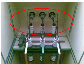
Figure 10 Evidence of water ingress at switchgear bushings.
